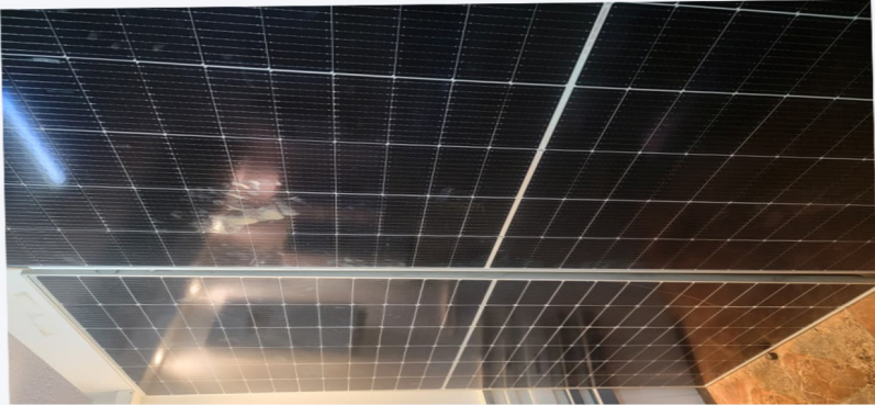
SOLAR PANELS SUPPLY
